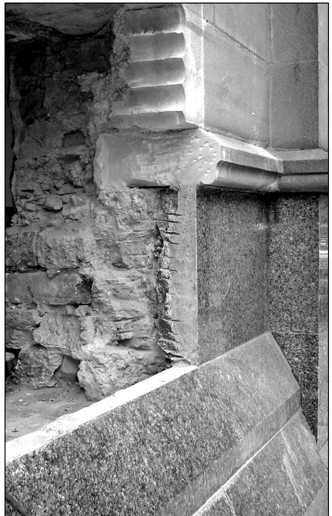
Figure 1. Cladding of sandstone, granite and larvikite, over the brickwork of the old Nottingham and Notts Bank (30), which was exposed during renovations in 2005.
